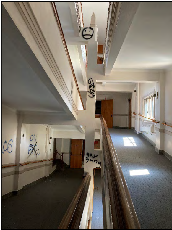
Fig. 55 – Main Building, interior, upper floor, main circulation ramps, longitudinal view and support column.
