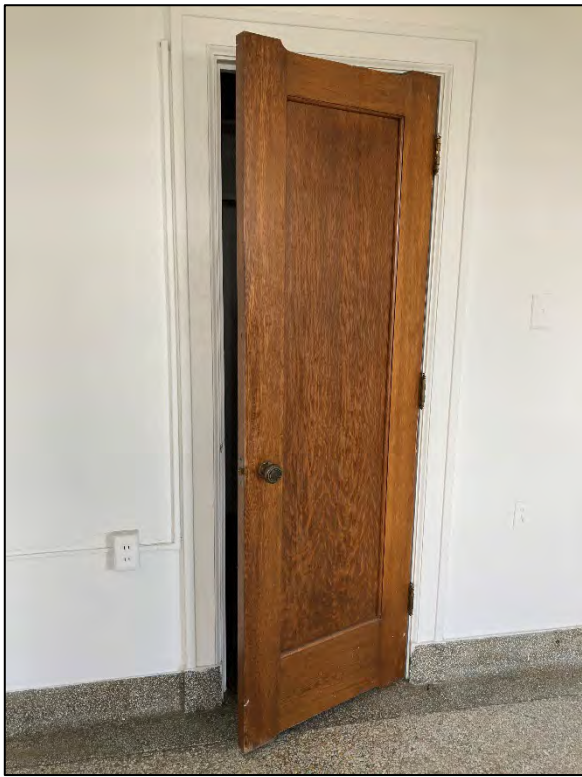
Fig. 71 – Main Building, interior, upper floor, typical residential unit, detail of closet door and trim.
