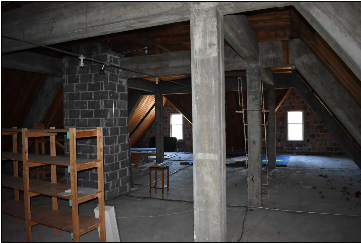
Fig. 65 – Main Building, interior, third floor attic space behind chapel/auditorium and above dormitory. (2019)
