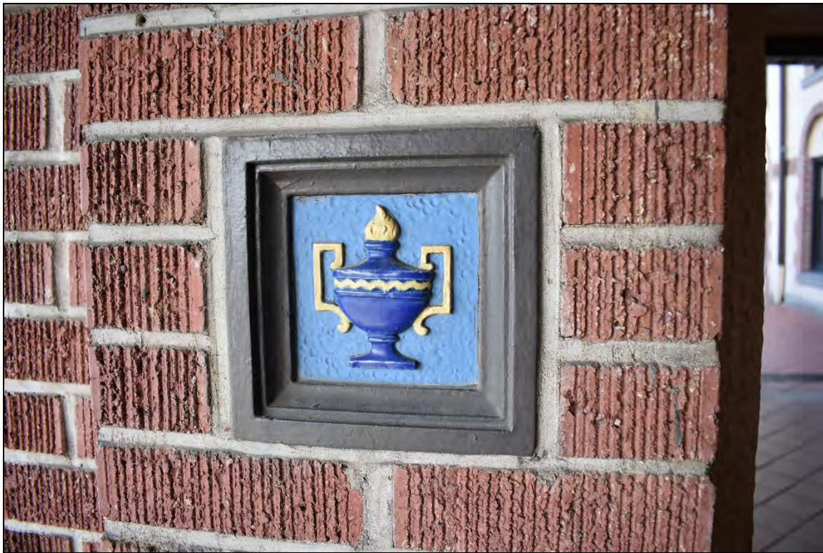
Fig. 8 – Main Building, west facade, main entrance porch, detail of Masonic ornamental tile.
