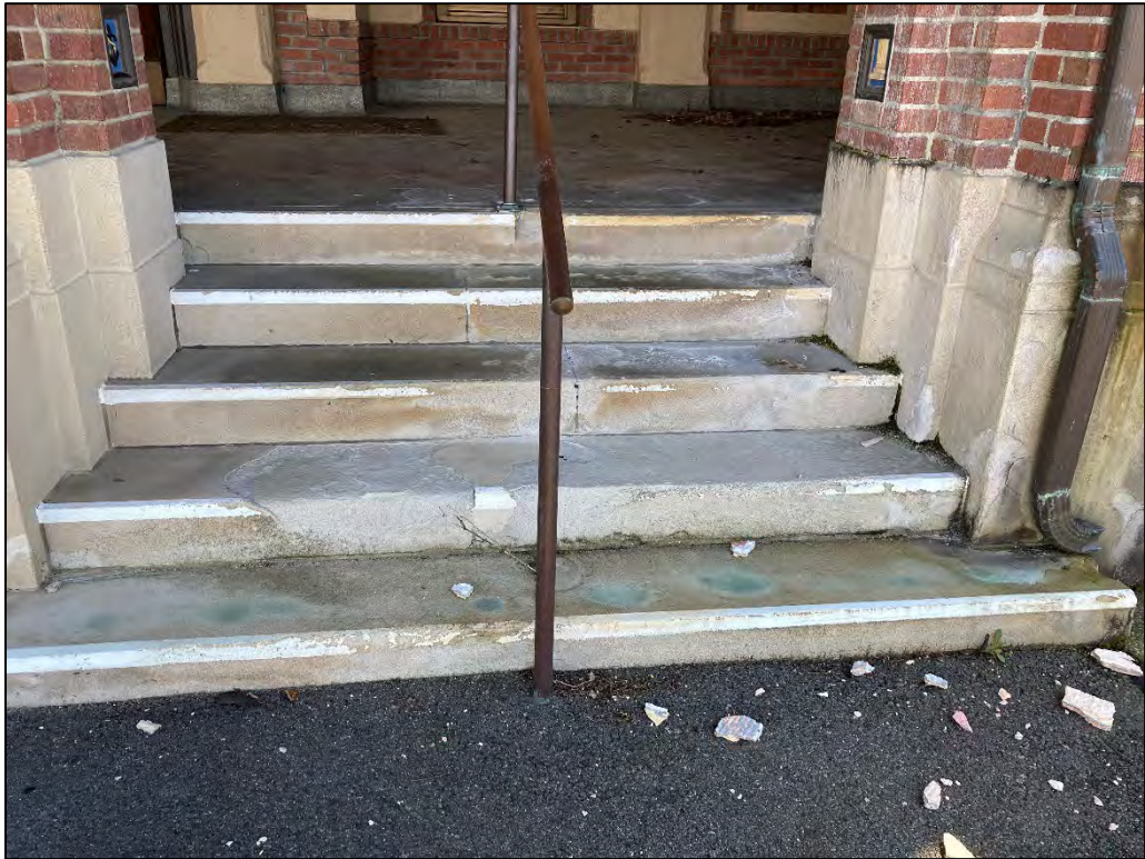
Fig. 38 – Main Building, front entrance steps, showing spalling and water damage.
