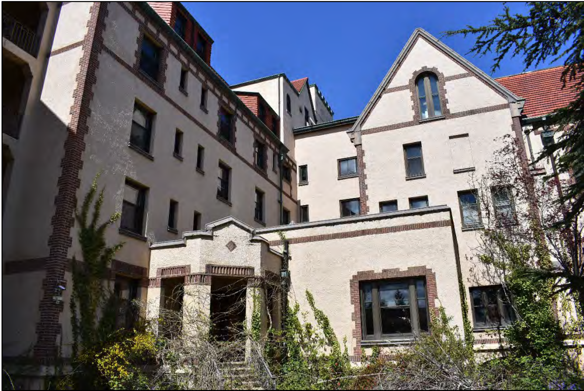
Fig. 21 – Main Building, south facade of rear wing (right) and east facade of south wing (left), from interior courtyard.
