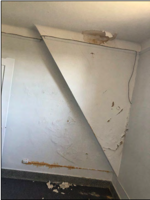
Fig. 88 – Condition: Main Building, interior, fifth floor, water damage.
