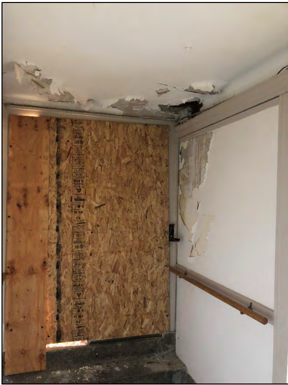
Fig. 87 – Condition: Main Building, interior, fifth floor, water damage at south wing.
