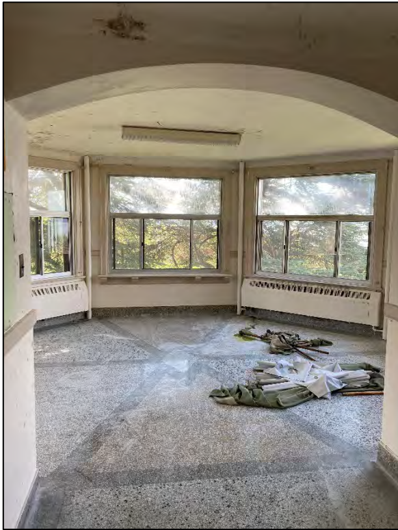
Fig. 72 – Main Building, interior, upper floor, typical solarium at end of residential corridor.
