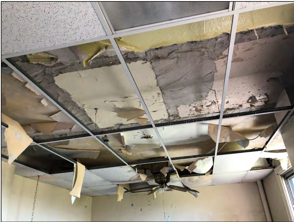
Fig. 81 – Condition: Main Building, interior, first floor, water damage at residence quarters.
