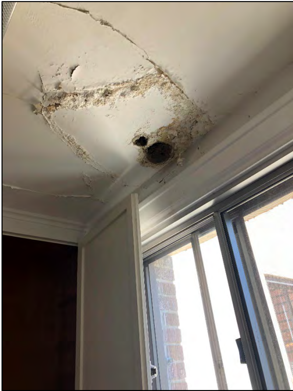
Fig. 84 – Condition: Main Building, interior, fourth floor, water damage at residential kitchen.
