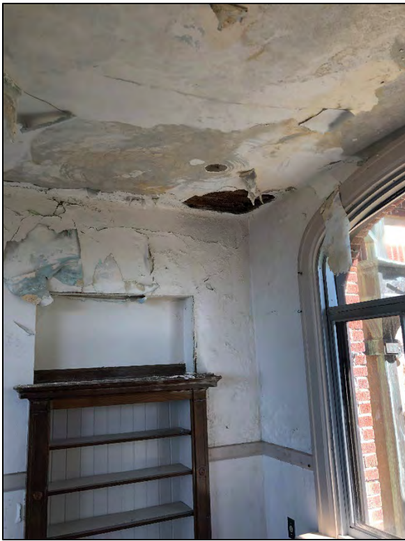
Fig. 85 – Condition: Main Building, interior, fourth floor, water damage at south Solarium.
