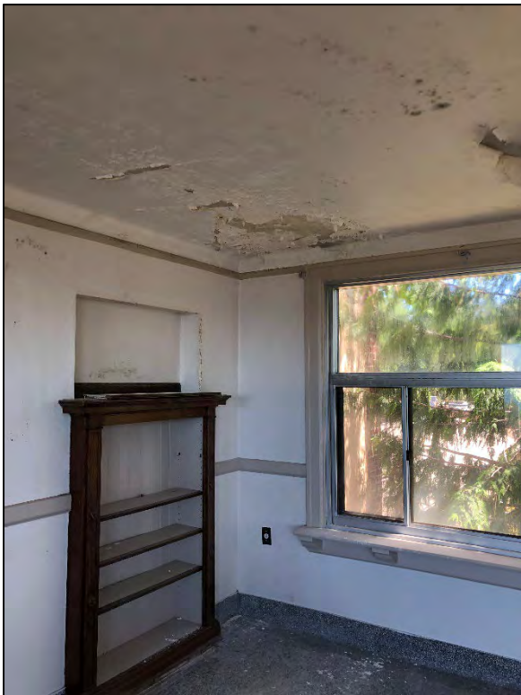
Fig. 82 – Condition: Main Building, interior, second floor, water damage at south Solarium.
