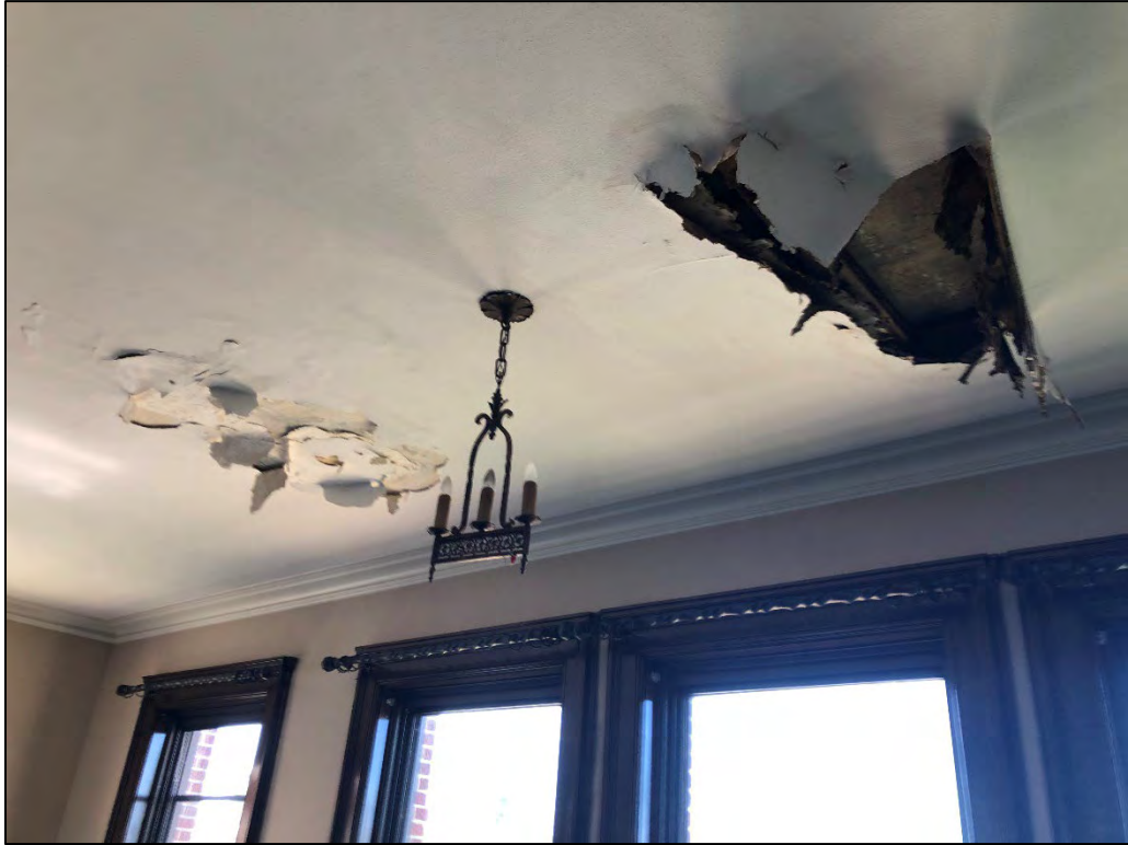
Fig. 80 – Condition: Main Building, interior, first floor, water damage at sitting room.
