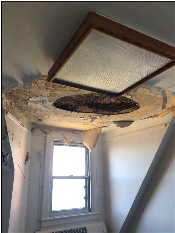
Fig. 86 – Condition: Main Building, interior, fifth floor, water damage at a bedroom.
