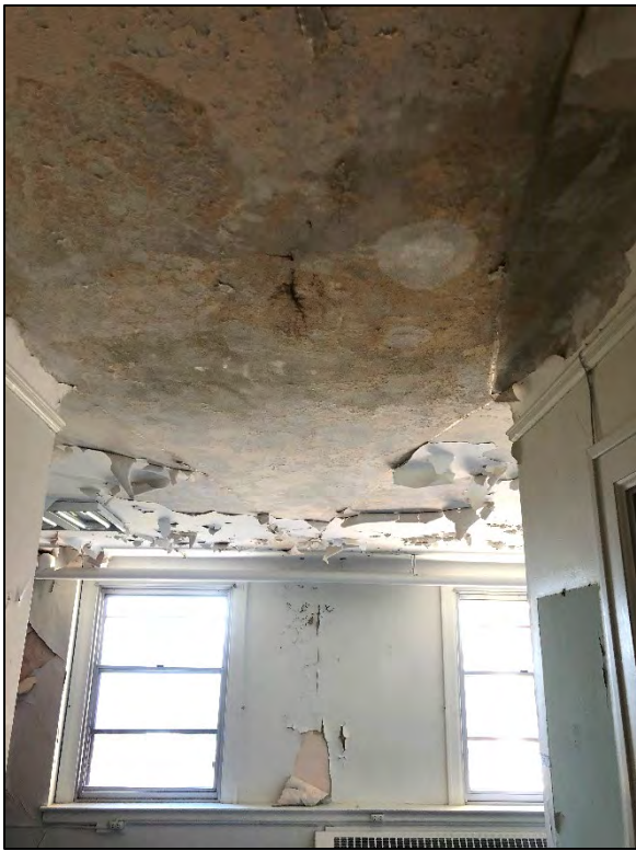
Fig. 83 – Condition: Main Building, interior, third floor, water damage.
